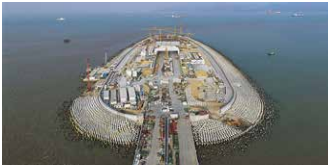
The tunnel section of the Hong Kong-Zhuhai-Macao bridge was completed on 7 July 2017, marking the end of construction of the main structure for the world's longest and deepest underwater tunnel
